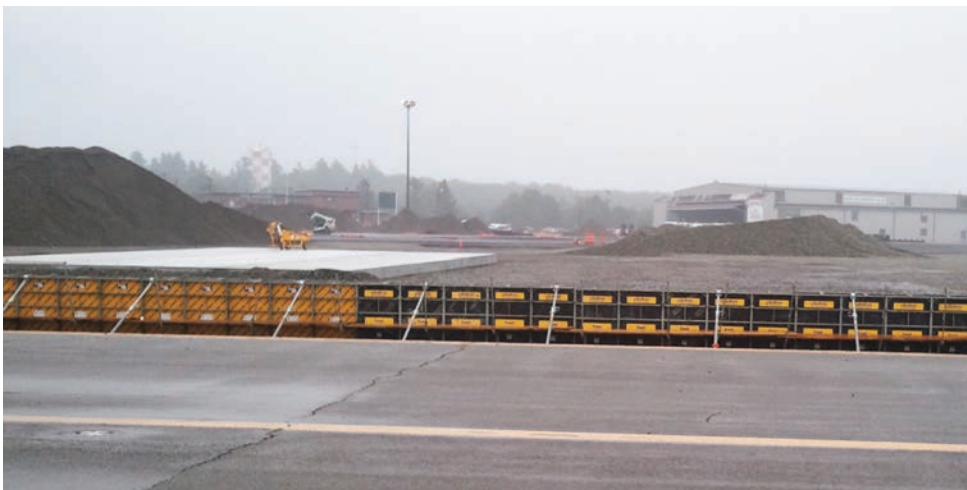
Below: Construction on the general aviation apron will be completed in October 2012
